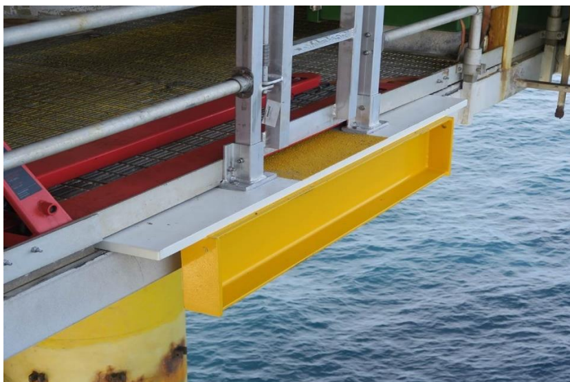
Figure 5 Landing area on the east side with platform installed. (Source: Aker BP)
